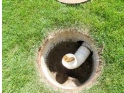
Figure- Concrete outlet vault with adjustable "swing joint" to control water elevation.
