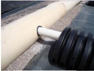
Figure- Inlet Header Pipe
