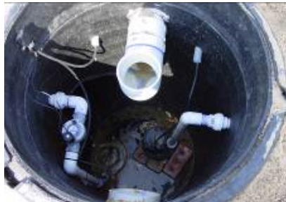
Figure - Reservoir access showing pump, float, & drain
