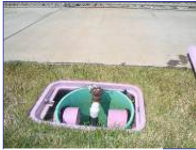
Figure - Inlet vault with gate valve inlet from pump in reservoir
